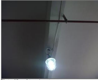
Photo of fire safety equipment explosion-proof light in warehouse.JPG
