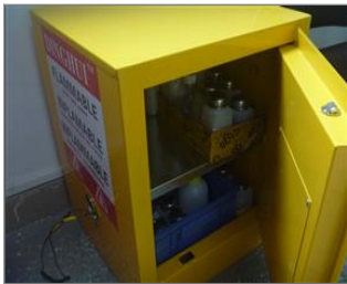
Photo of chemical storage room (if applicable) cleaning solvent stored in a anti-leakage cabinet.JPG
