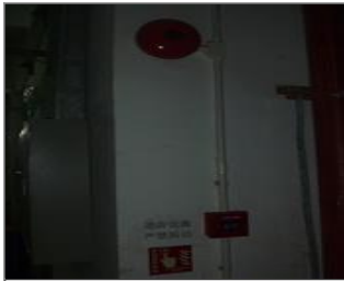
Photo of fire safety equipment fire alarm.JPG
