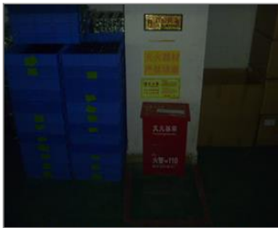
Photo of fire safety equipment fire extinguishers.JPG
