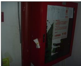
Photo of fire safety equipment fire hydrant.JPG
