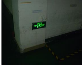
Photo of fire safety equipment lighting evacuation arrow.JPG
