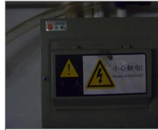
Photo of fire safety equipment Corrected for last audit-warning sign posted on electric control station.JPG
