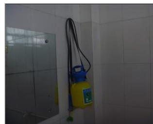
Photo of the personal protection equipments (if applicable) eye washing facility.JPG
