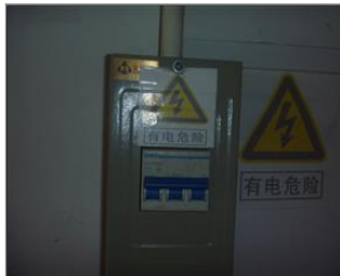
Photo of non-conformity NC-electrical switch box was without outer cover.JPG
