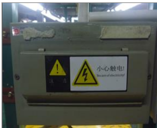
Photo of fire safety equipment electrical switch box with outer safety guard and shock warning sign.JPG
