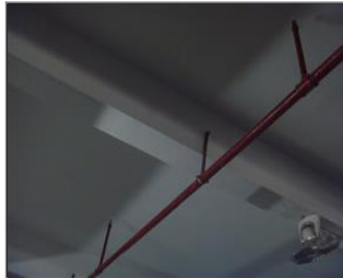
Photo of fire safety equipment sprinkler.JPG
